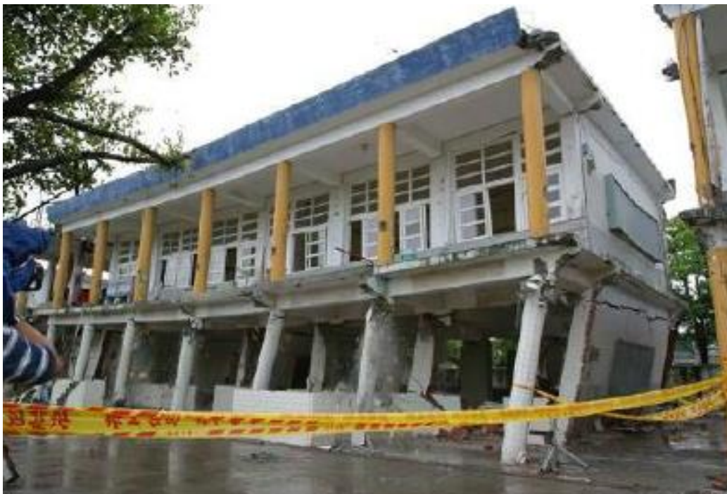
Figure 5. The deformed school building after the traditional pushover test (Kouhu Elementary School, Yunlin, Taiwan) (Zhong, et al. , 2013).
