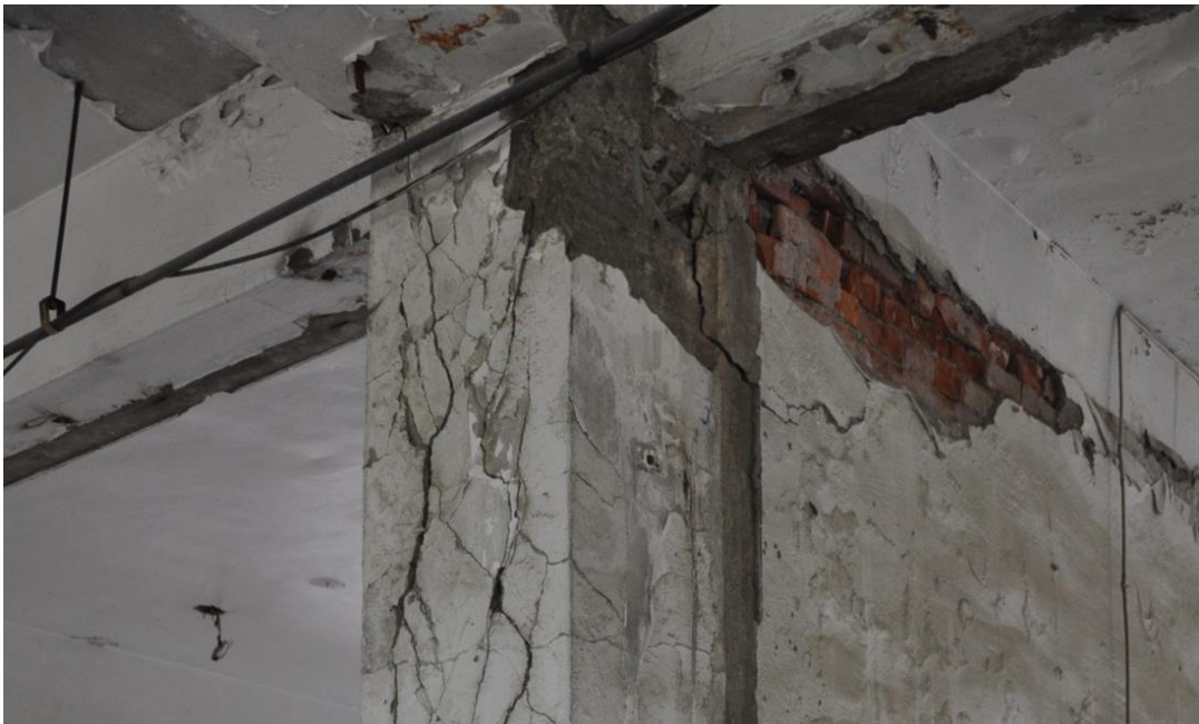
Figure 15. Cracks at the joint of a column and girder during an earthquake.
