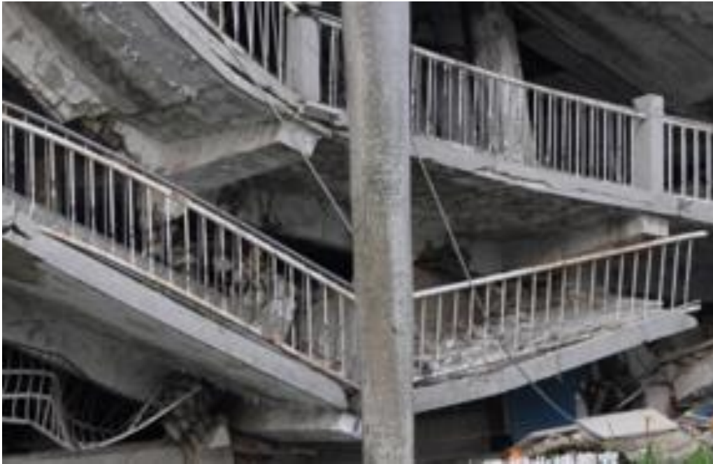
Figure 16. Break in the joint of a column and girder after an earthquake.
